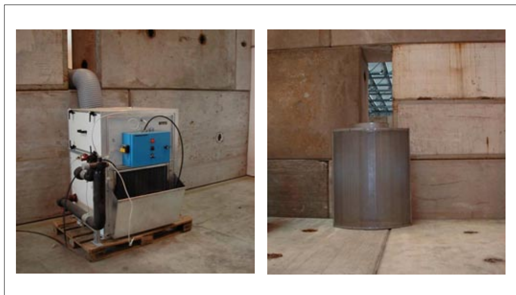
Figure 5.4 Supply fan and diffuser
