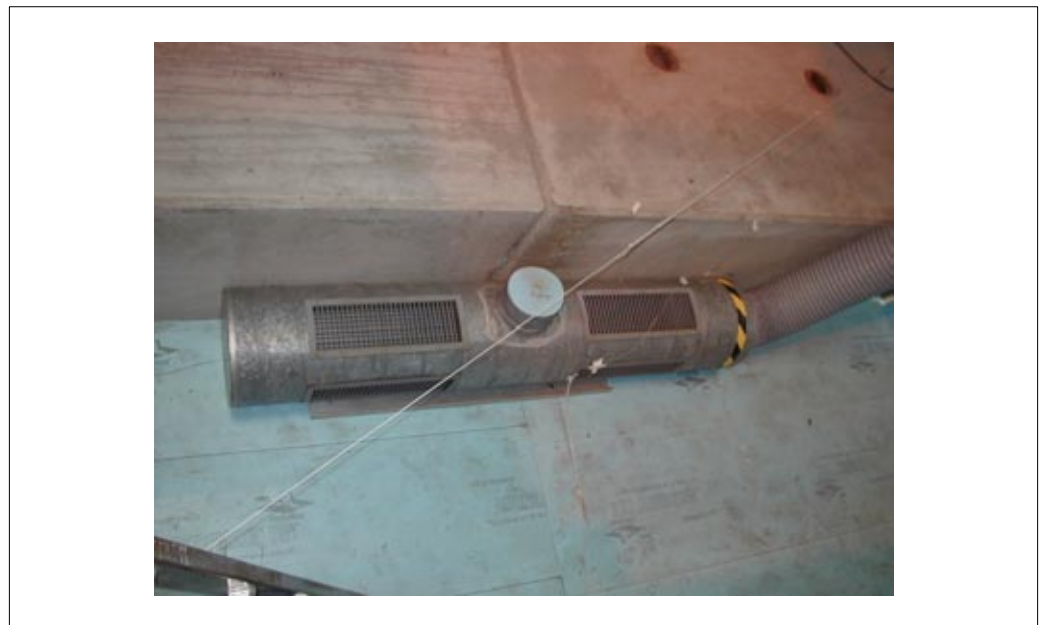
Figure 5.5 Extraction diffuser in the pit
